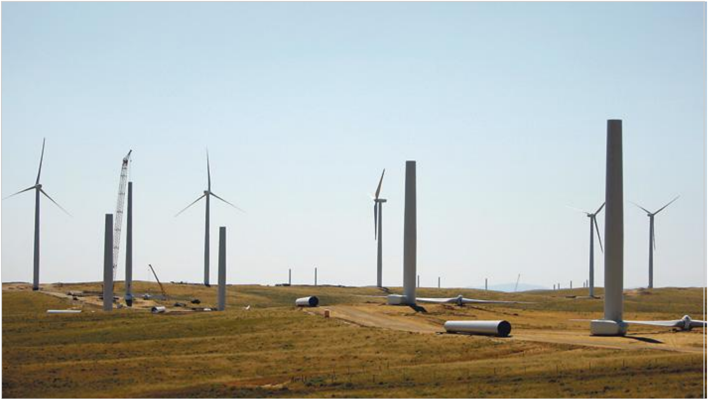
A wind farm is shown under construction near Glenrock in this file photo from August. (Dan Cepeda/Star-Tribune)
