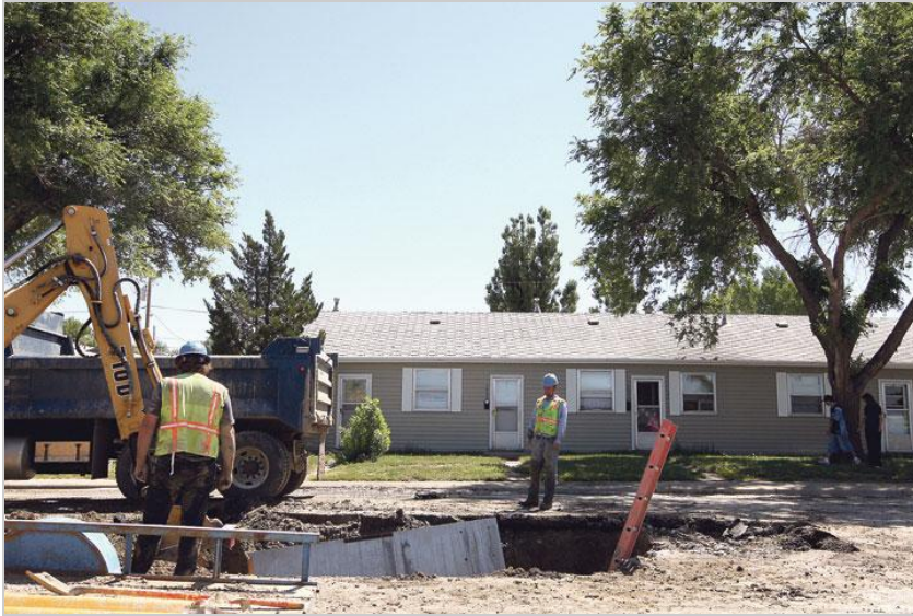
A crew works to fix a 12-inch water-main break in the 1000 block of Beverly Street on Wednesday. Officials hoped to restore water service before Wednesday afternoon, but the road will be closed through today so the road can be fixed. (Kerry Huller/Star-Tribune)
