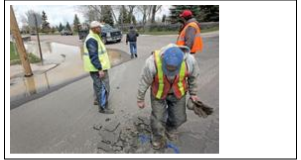
City workers turn off the water at the corner of Ninth and Canby streets last spring after a water main under the intersection broke. Boomerang file photo
