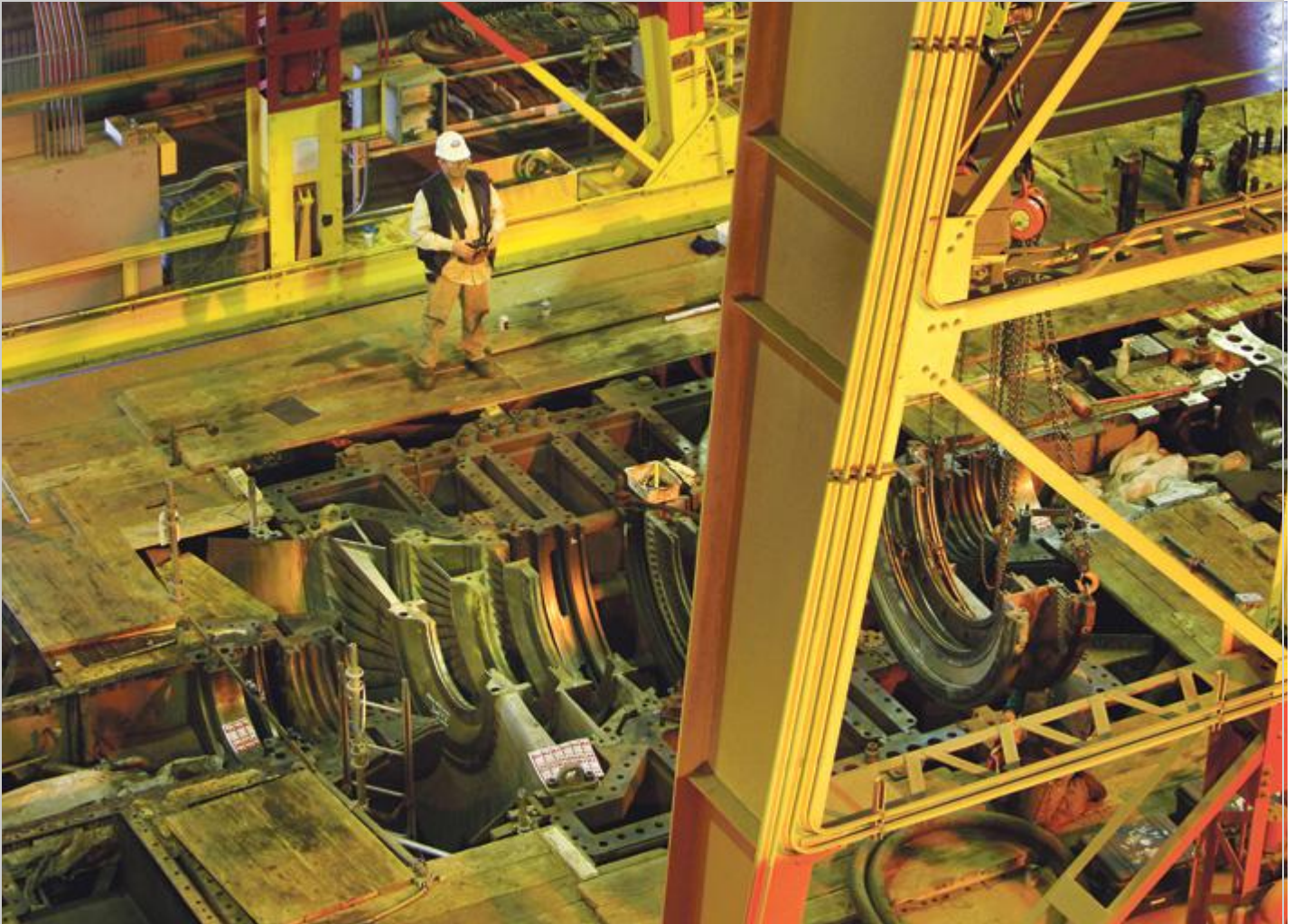
Workers disassemble one of the power generators during an overhaul project at the Rocky Mountain Power's Dave Johnston Power Plant in Glenrock. The massive maintenance overhaul and expansion project is keeping hundreds of contract employees employed. Photo by Dan Cepeda, Star-Tribune
