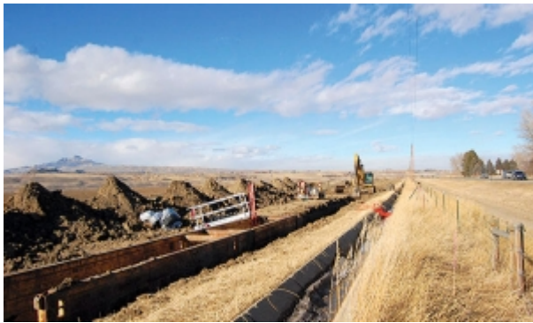
In a trackhoe, Garney Wyoming employee Kyle Sweat backfills a ditch for the Shoshone Municipal Pipeline to relocate about 2.5 miles of pipe further from U.S. 14-A, thus allowing space for Wyoming Department of Transportation's project to widen the highway. Tribune photo by Gib Mathers
