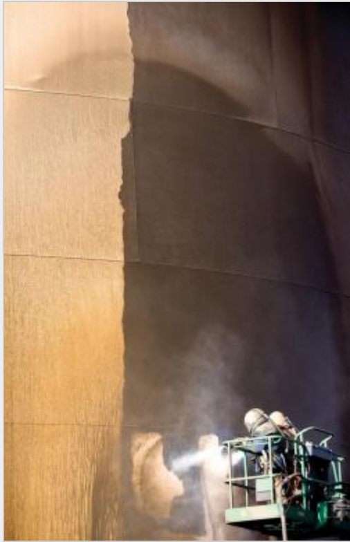
Workers from State Painting of Utah blast the paint off of the outside of a water tank in the Foothills neighborhood. The company was hired by the city to strip paint from the outside and inside of the tank and paint the metal vessel. - News-Record photo by Nathan Payne
