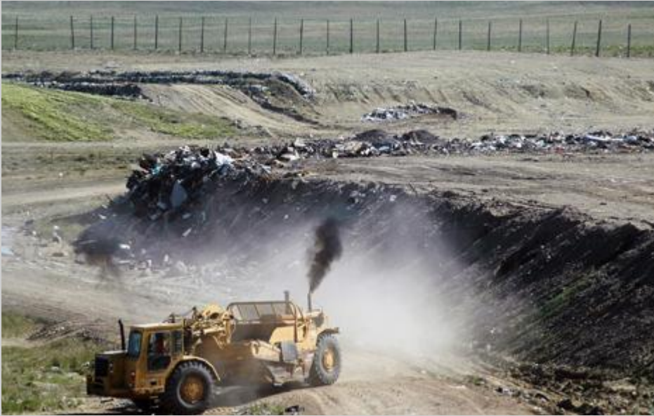
(Rawlins Daily Times, Kathy Johnson) The scraper at the Rawlins Municipal Landfill pulled up onto one of the facility's main roads on Tuesday morning.
