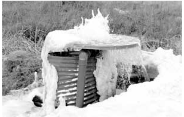
The in-stream air stripper, located near Missile Dr. and South Creek Dr. The stripper cleans the water of a hazardous degreaser and sometimes emits water into the air. / Courtesy Photo
