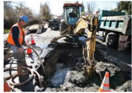
ANDY CARPENEAN/Boomerang photographer Dennis Skinner, a city of Laramie water maintenance worker, uses a hose for a sump pump to drain the water from the hole where a water main broke at 13th and Steele Thursday. The break was one of three water main breaks in that area of town.
