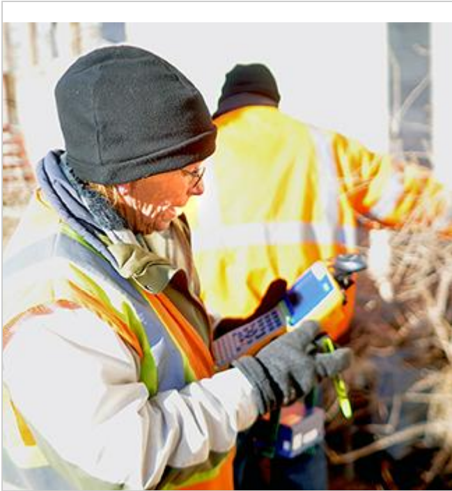
(Rawlins Daily Times, John Feely) Rawlins meter reader Becky Strand checks her equipment Tuesday while co-workers install a radio read transmitter on the water meter at the Victory Baptist Church on West Cedar Street.
